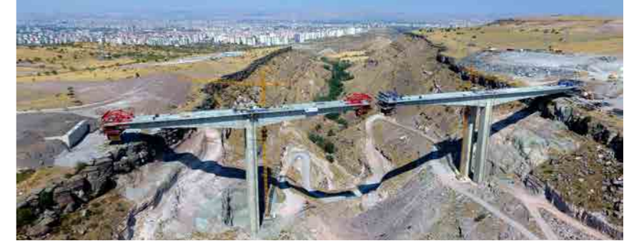
Kayseri Derevenk Viyadüğü Dengeli Konsol-Ardgerme. Kayseri Derevenk Viaduct Balanced Cantilever and Post-Tensioning works.
